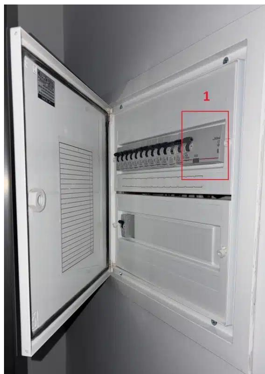
Laundry fuse box
